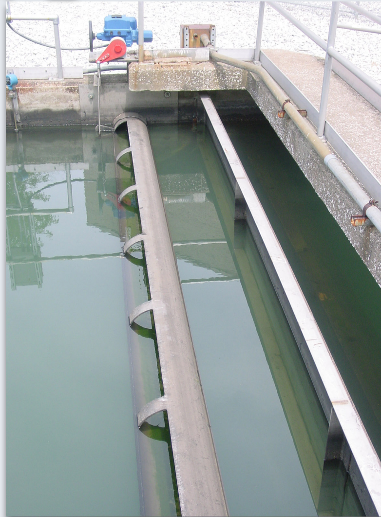
Slotted Pipe in Tank of Untreated Water
